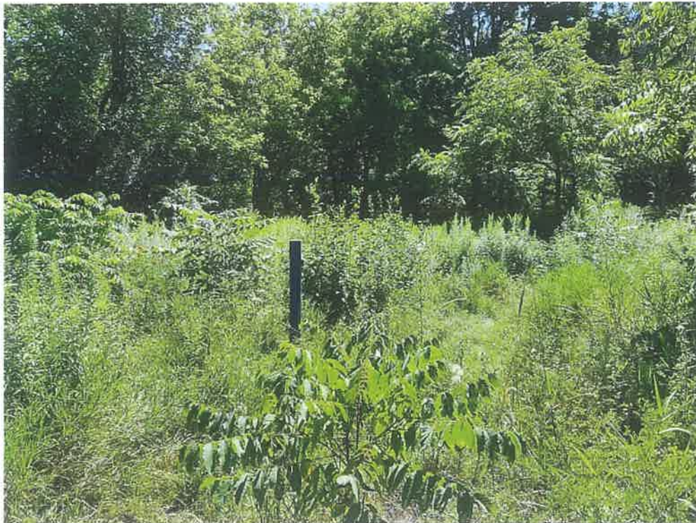
A view of a monitoring well located in the southwest portion of the subject site (looking east)
