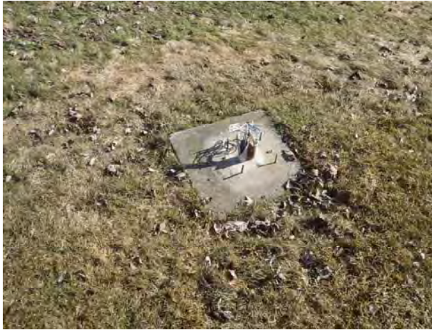
Plate 13: Former light standard base with wiring.
