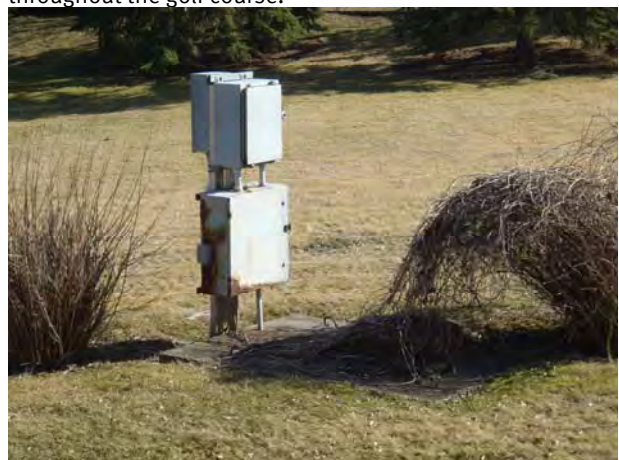
Plate 12: Buried utilities consisting of a transfer box and manhole cover located within the golf course.
