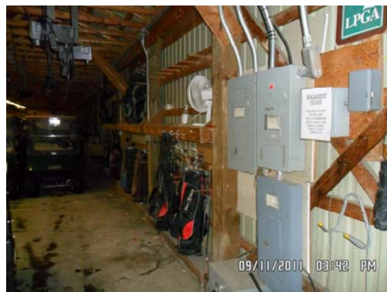
Photo 6: Golf cart storage area with transformers and old golf equipment
