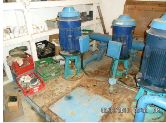
Photo 8: Pump house with sump
