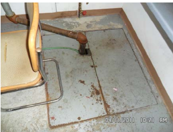
Photo 5: Sump in sprinkler room in clubhouse
