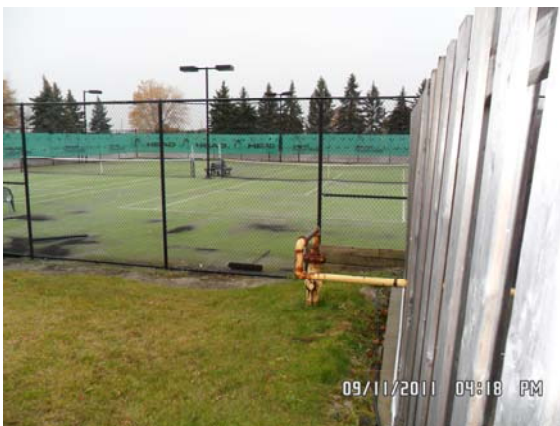
Photo 11: Natural gas pipeline entering Site
