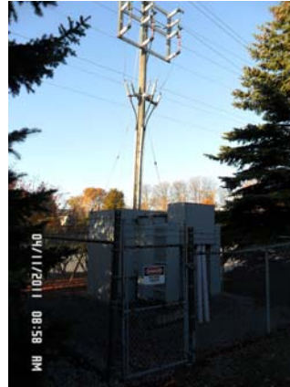
Photo 2: Large outdoor transformer
