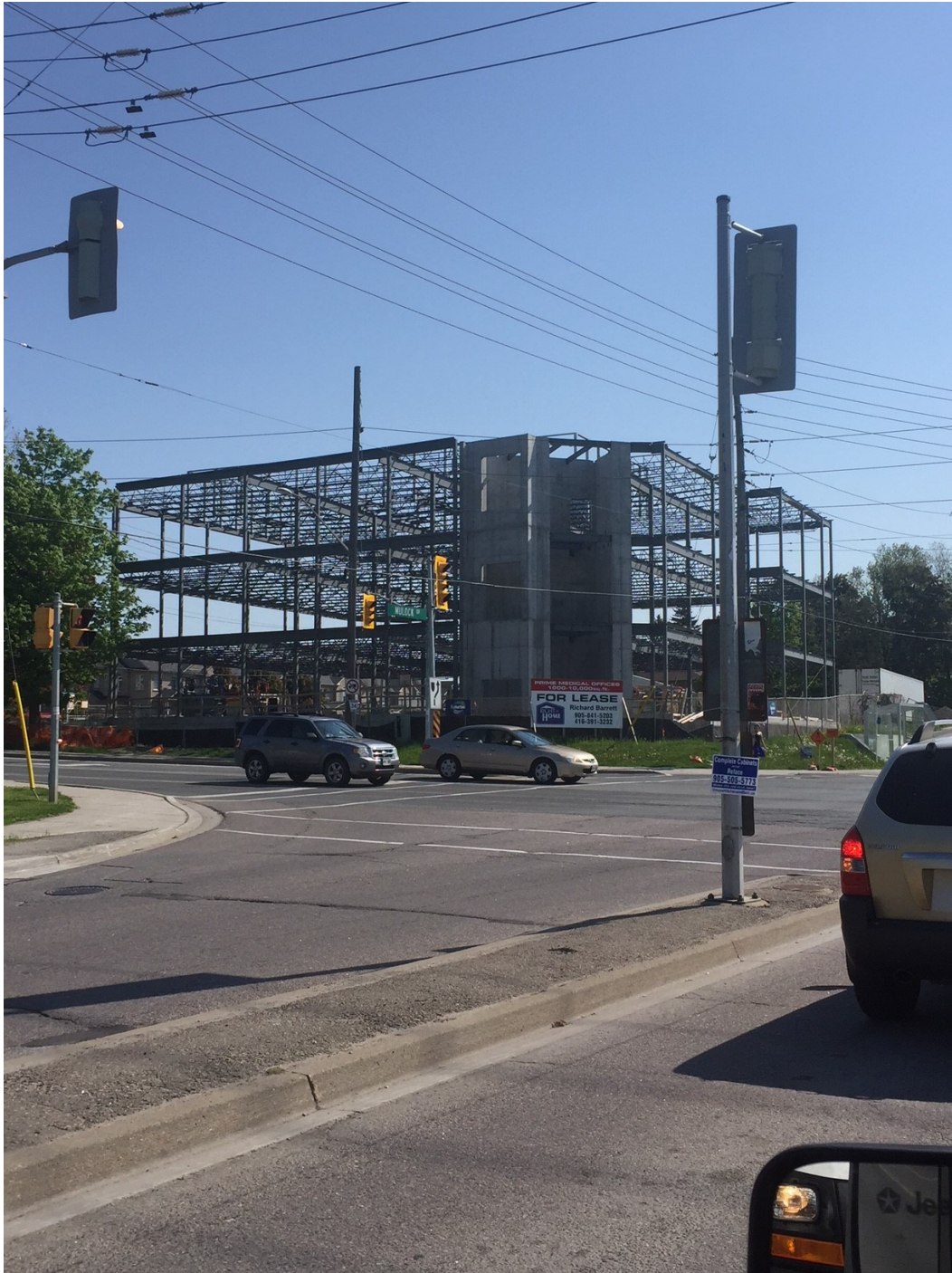
New medical services/offices use under construction at 536 Mulock Drive (north east corner of Mulock Drive and Bayview Avenue)
