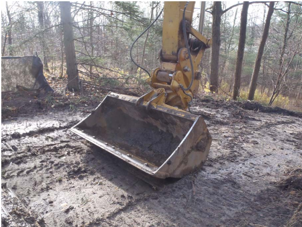
Photograph 2: Contaminated topsoil removed with smooth bucket to control interface with underlying soil.
