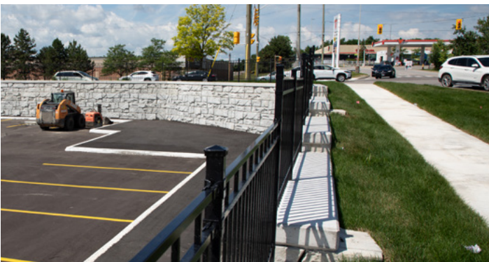
Retaining walls and decorative fencing prevent erosion, provide barriers and create an attractive roadway.
