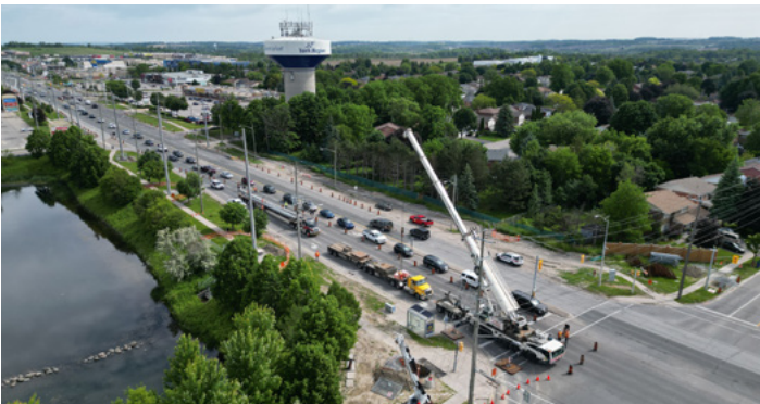
Through a partnership with NT Power, 68 hydro poles were installed along the two-kilometre corridor.
