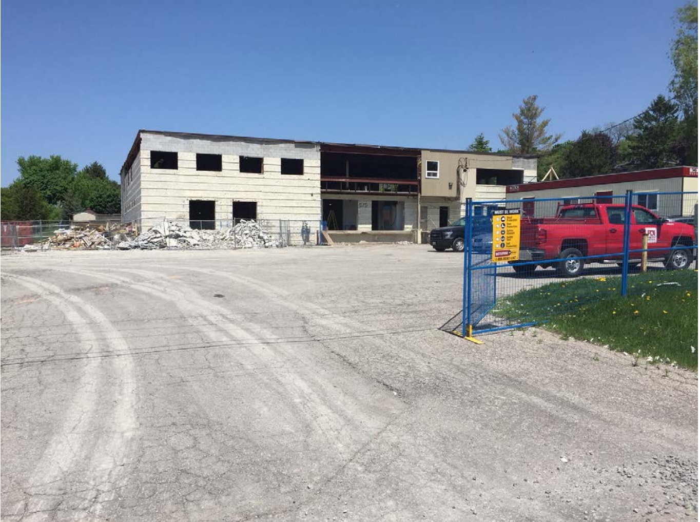
New human services agency use (Community Living Central York) under renovation at 575 Penrose Street (north west of Mullock Drive and Bayview Avenue)
